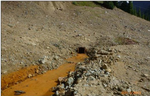
Figure 7.—Photograph showing the seepage outflow from the drain pipe at the American Tunnel at Gladstone, Colorado, as it appeared on September 3, 2015, with about 100 gpm of acid water flowing out.
