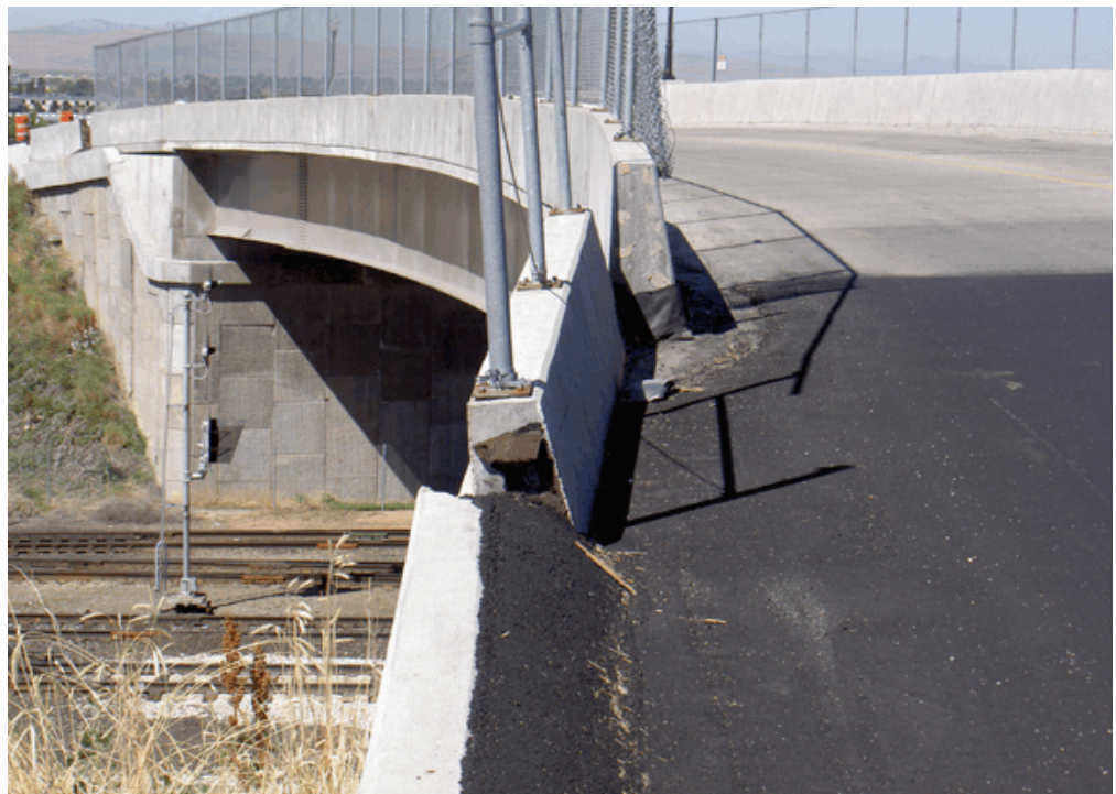
Figure 3.5 Failed Ramps on Bridge on 200 South in Clearfield City. The designs for the 200 South bridge in Clearfield were changed in order to reduce costs, and the materials used did not meet specification. As a result, the ramps to the bridge began to sink a week after the bridge was opened.
