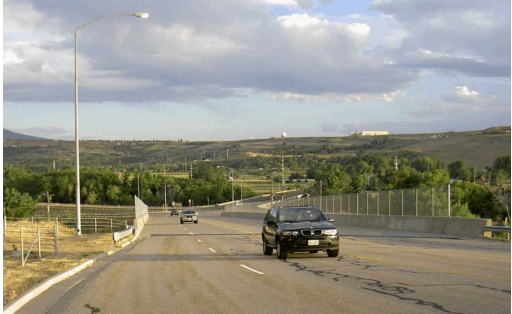
Figure 3.2 Bridge over Adams Avenue Lacks Shoulder for Emergency and Pedestrian Use. UDOT engineers indicated that their standards require that the bridge include enough width for a shoulder on each side of the road.
