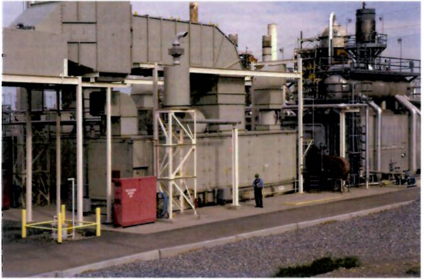
The CHP system operates efficiently and reliably 24/7 and supplies all of the refinery's power and steam needs, with excess power sold to the grid.
