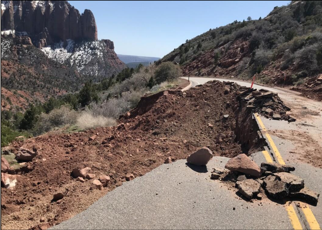
April 2023 Kolob Canyon Rockfall/Landslide
