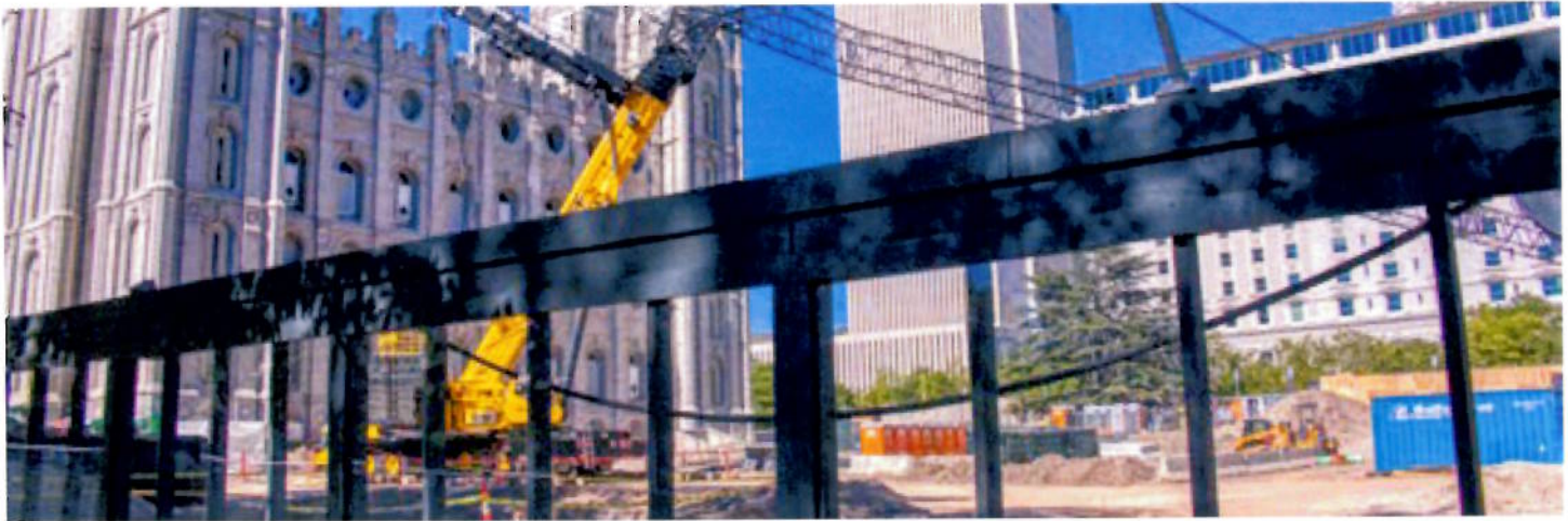
The Salt Lake Temple is currently undergoing a major seismic upgrade to prepare for the “Big One.”
