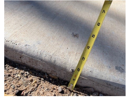
Transition from parking to sidewalk that is too abrupt.
